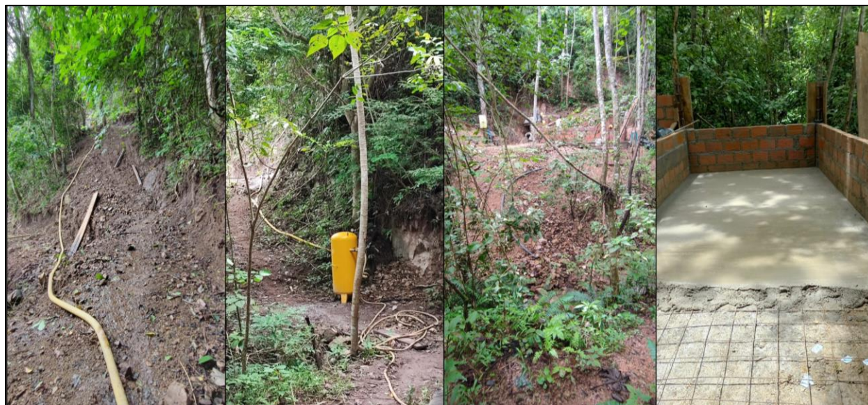
Photo 1. Access road and construction of ancillary mining infrastructure at the Mariana Mine.
